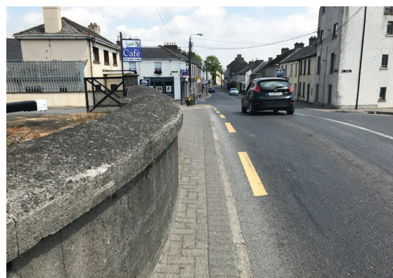
Figure 2.38: Substandard footpath on Augustus Bridge
