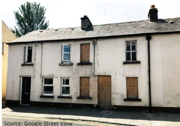
Figure 2.24: Derelict houses on Offaly St. (August 2018)
