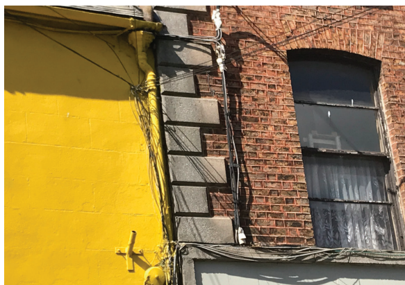
Figure 2.32: A proliferation of wiring on Leinster Street
