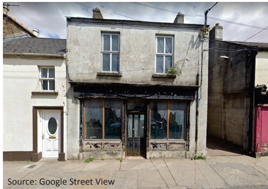
Figure 2.26: Derelict unit on Offaly St. (August 2018)
